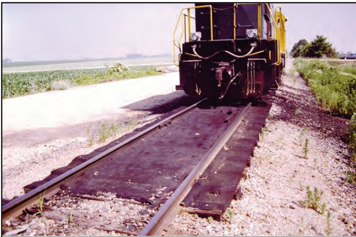
Track mat on the Illinois RailNet north of Flagg Center where the locomotive is parked when not in use.
