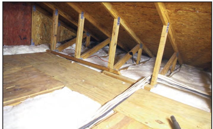
The insulated attic. It had lots of boards to crawl on. Electric wires in Florida are not in conduit.
