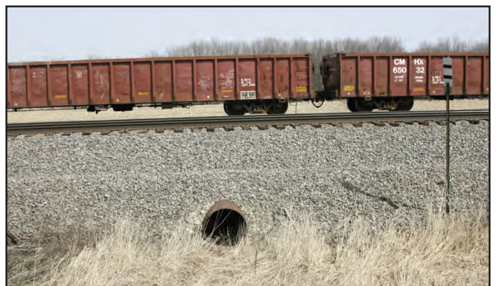
Culvert is several feet below the ties. CN at Duplainville, WI.
