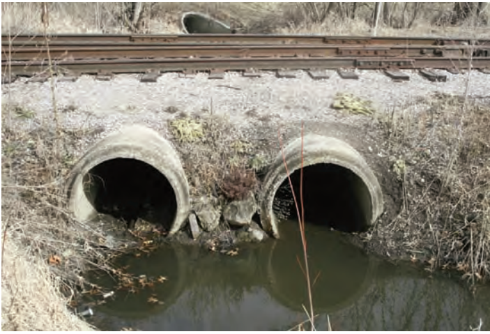
Spring runoff fills the drainage ditch below the culvert. Canadian Pacific at DeForest, WI.
