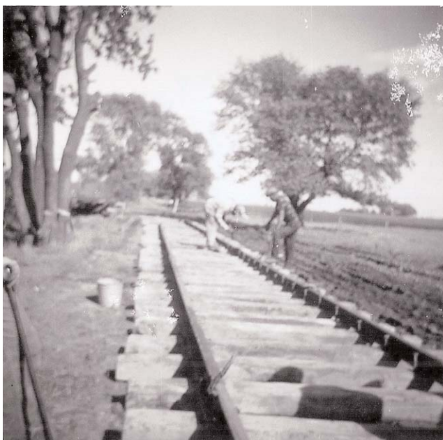
Bob Bruneau working on the right of way, putting down rail in anticipation of the equipment.
